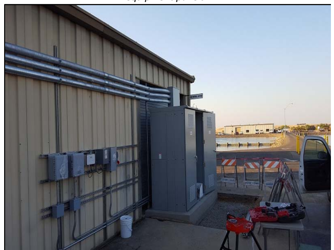
Photo of new switchgear and breaker panel and SMUD monitoring equipment panels.
