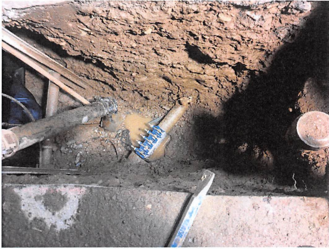
Photo 4: Temporary repair at break dated 12/12/18.
