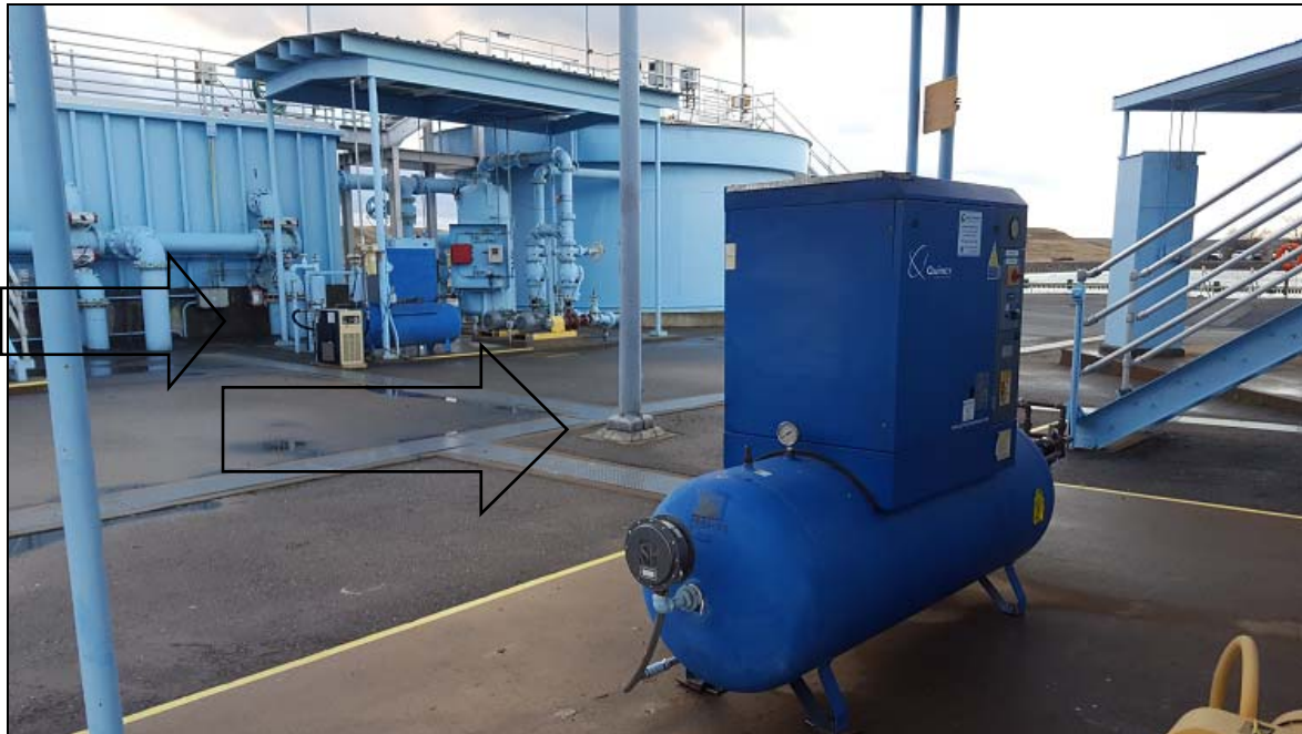
Photo of existing compressors at Wastewater Reclamation Plant
