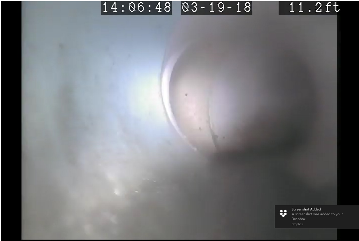
Capture #14: Beyond area of failure toward sewer main (further)
