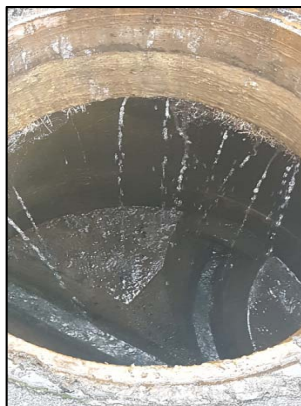
Manhole with I&I
