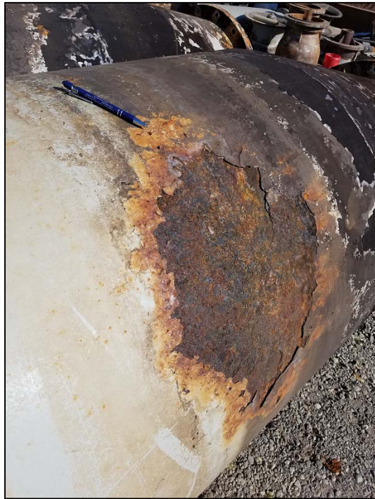
Corrosion of pipe column
