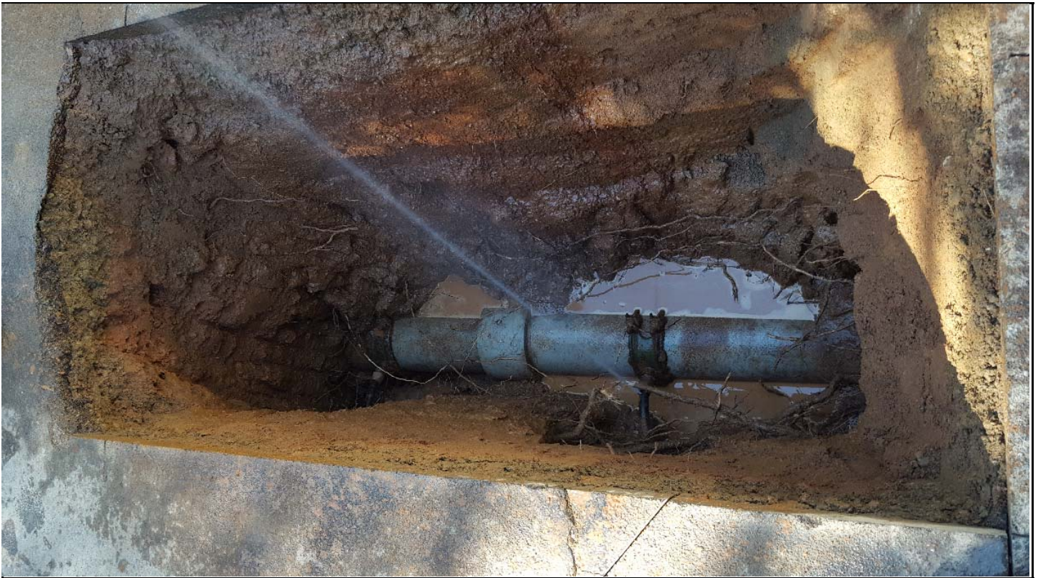
Water service line leaking near connection to water main – Puerto Drive
