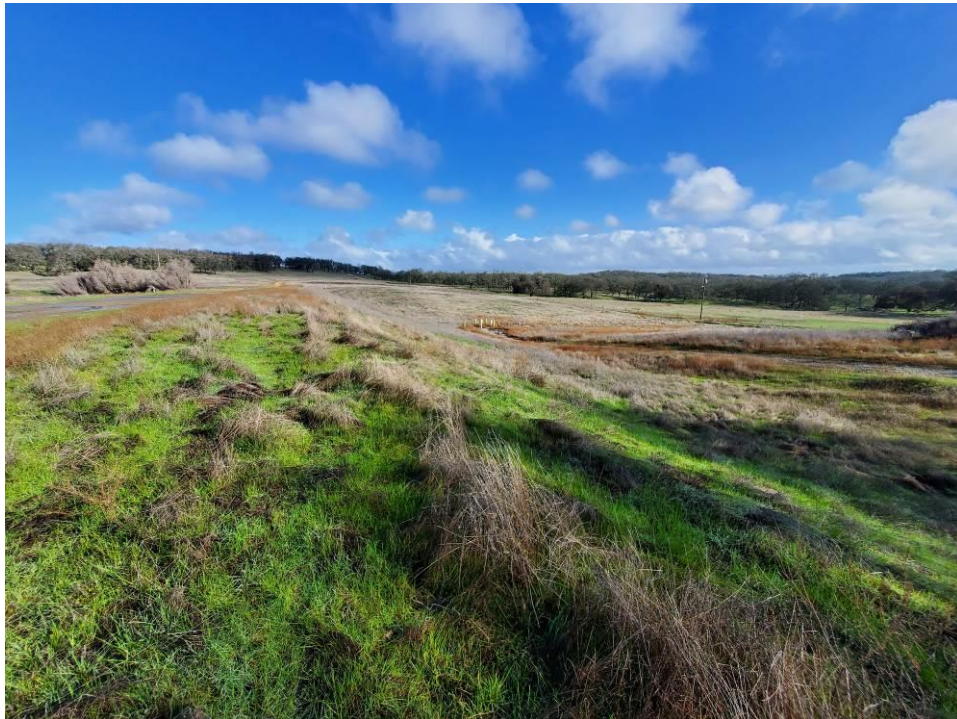
Photo 4: View of the downstream face of the East Dam from near the right abutment looking towards the left.
