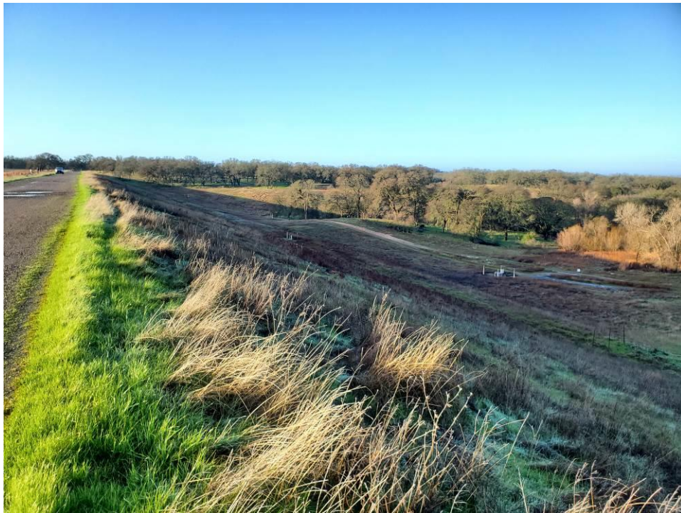
Photo 2: View of the downstream face of the Main Dam from near the right abutment looking towards the left.
