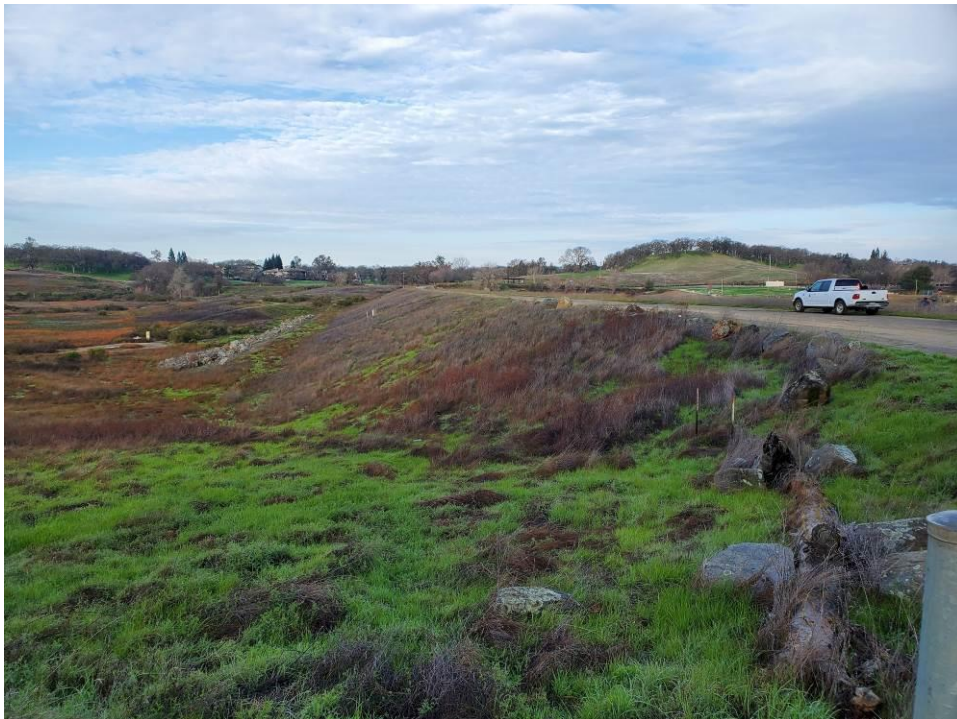
Photo 2: View of the downstream face from near the left abutment looking towards the right.
