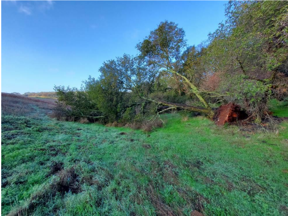
Photo 5: View of the downstream face of the Main Dam near the middle of the dam. The fallen oak tree in this location needs to be removed.
