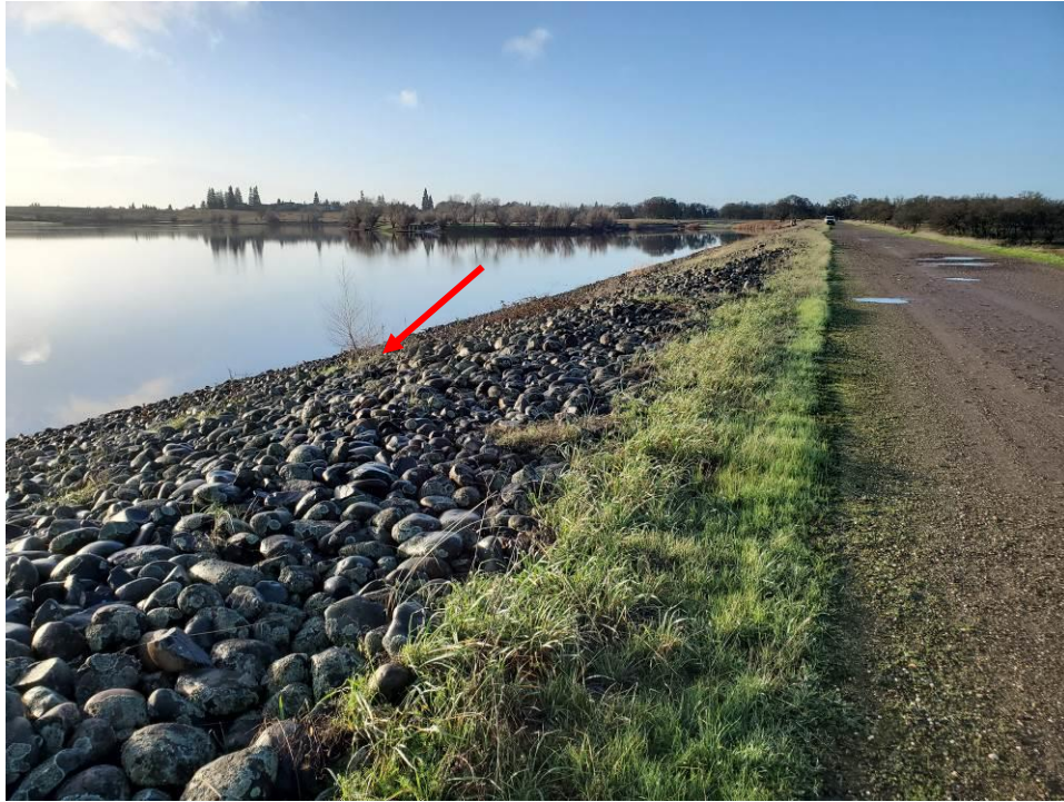
Photo 1: View of the upstream face of the Main Dam from near the right abutment looking towards the left. The small tree shown by the red arrow needs to be removed.
