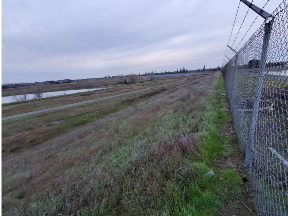
Photo 1: View of the downstream face and toe on the west side of the ponds.
