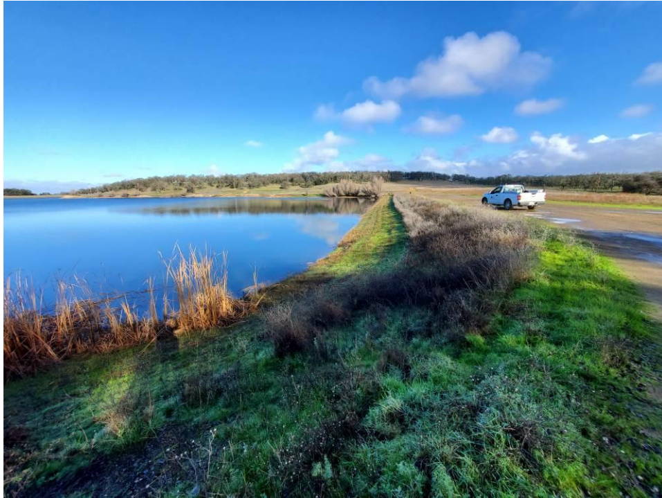
Photo 3: View of the upstream face of the East Dam from near the right abutment looking towards the left.
