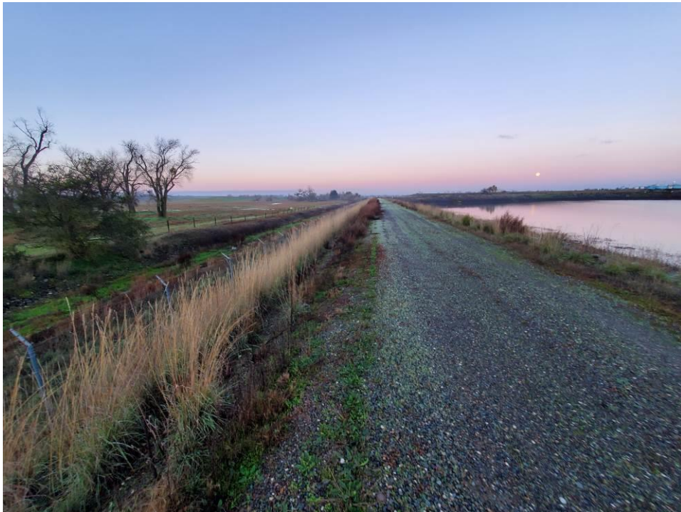
Photo 2: View of the south side crest and downstream face of the dam at Reservoir No. 1 looking west.
