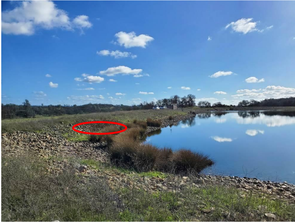
Photo 1: View of the upstream face of the Middle Dam (near) and South Dam (far) from the left side of the Middle Dam looking towards the right. The berry vine growth in the red circle needs to be removed.
