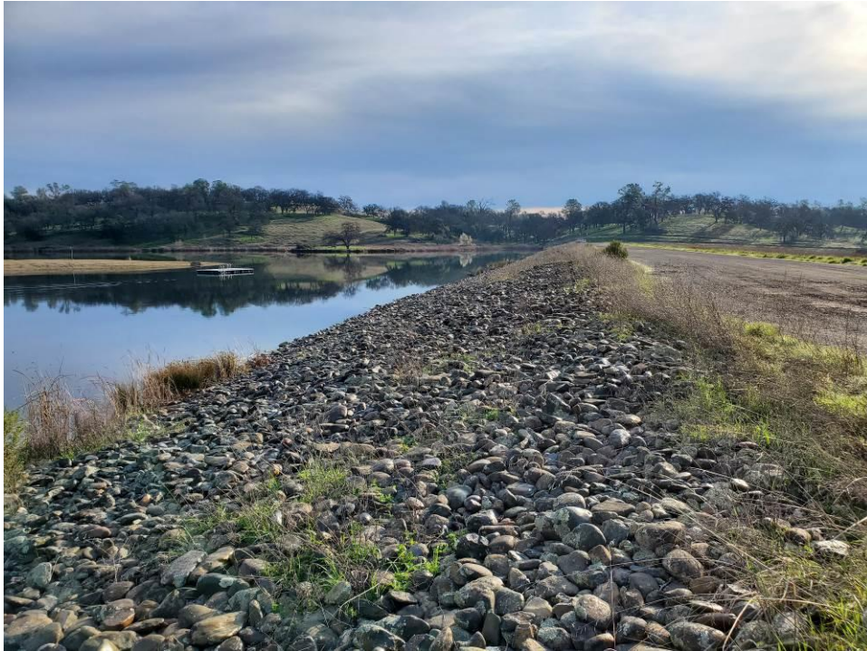
Photo 1: View of the upstream face from near the right abutment looking towards the left.
