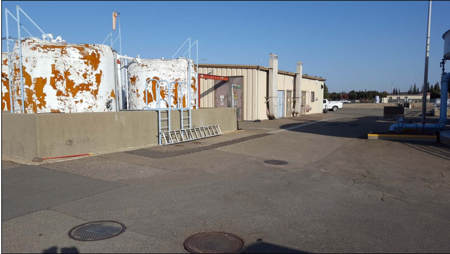
View of bulk chemical tanks, trench, and control building at tertiary treatment facility
