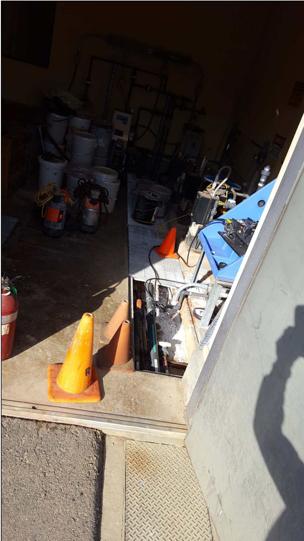
View of chemical feed room and piping trench
