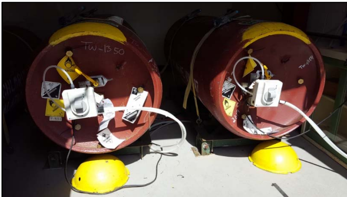
Existing Chlorine tons and feed system
