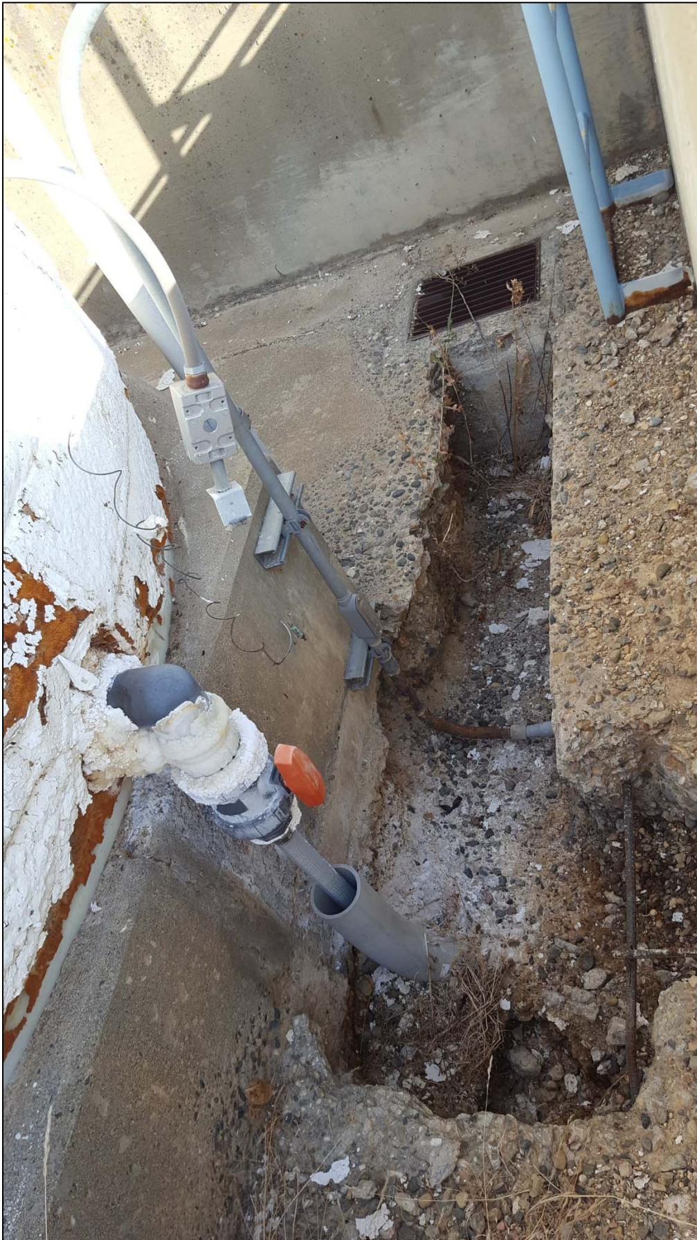
View of discharge from existing caustic tank
