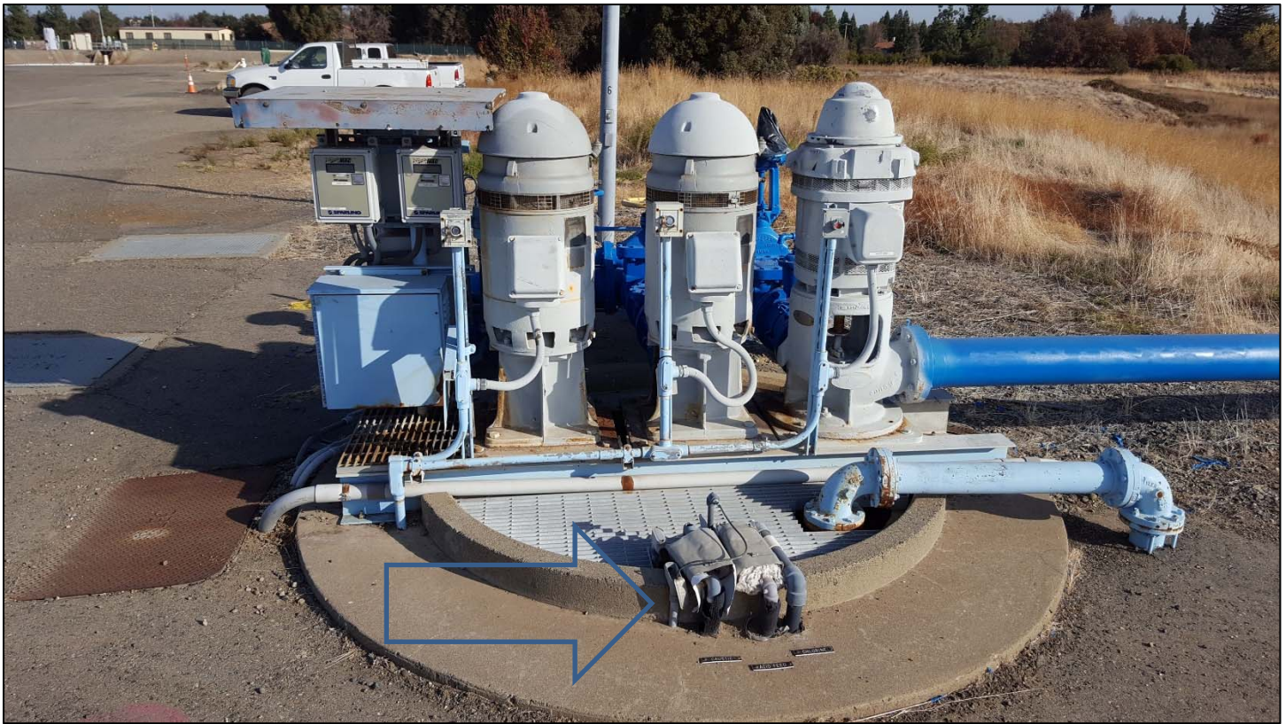
Tertiary pump station with chemical feed lines feeding into wet well
