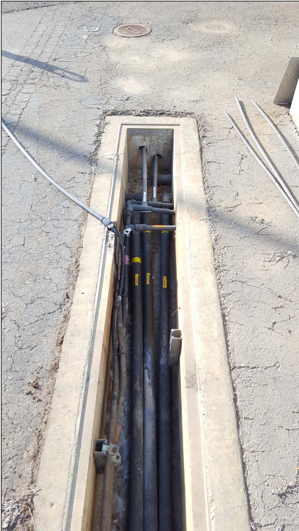
View of chemical piping trench towards tertiary pump station
