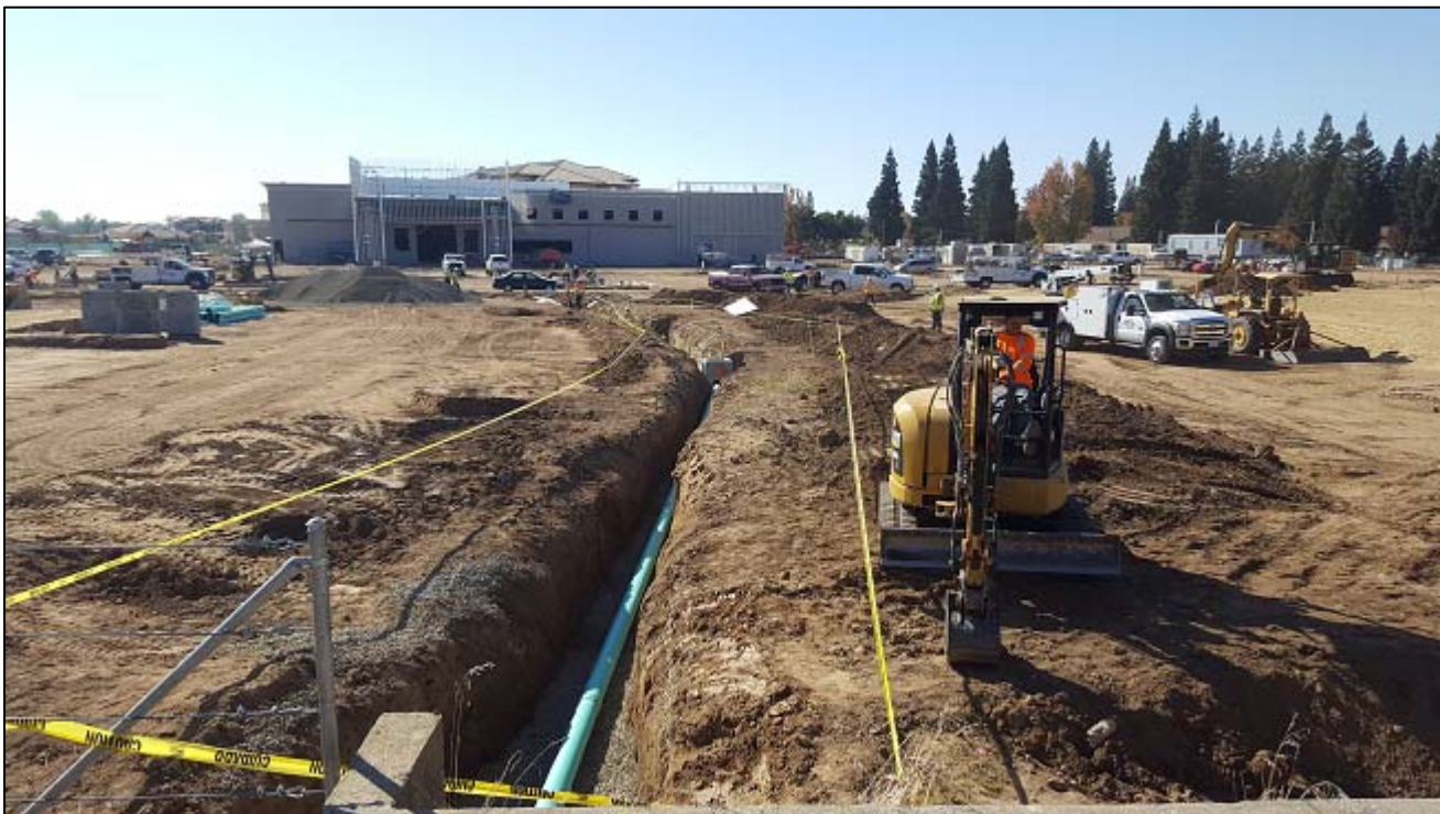
View of storm drain line being installed between lots 4 & 5 with future BelAir in the background
