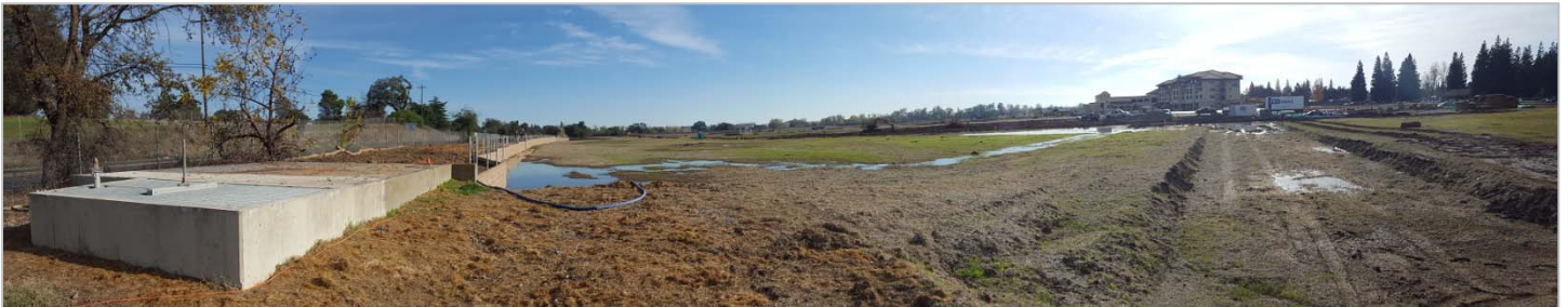
Photo of the CIA Ditch diversion structure after a section of it being lowered with Marketplace site and Inn in the background
