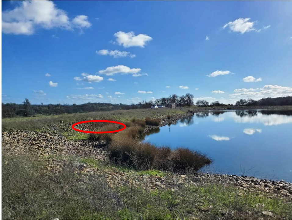
Photo 1: View of the upstream face of the Middle Dam (near) and South Dam (far) from the left side of the Middle Dam looking towards the right. The berry vine growth in the red circle needs to be removed.
