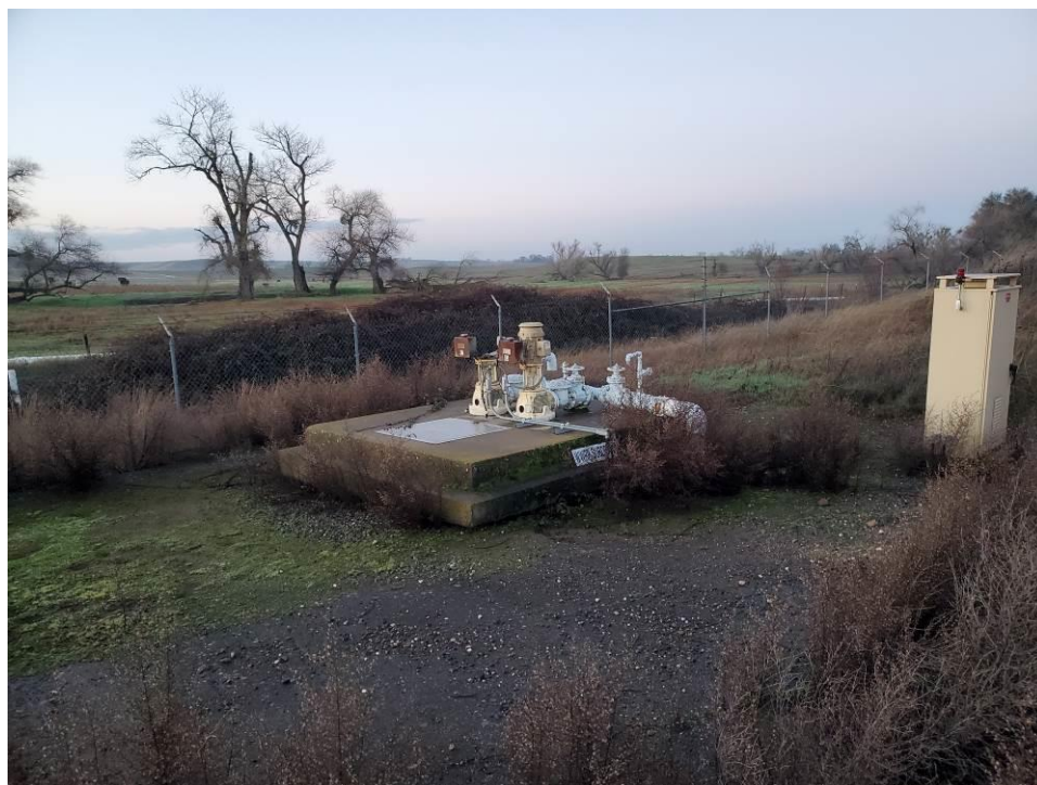
Photo 3: View of the reservoir dewatering pumps located at the southwest corner of Reservoir No. 1.
