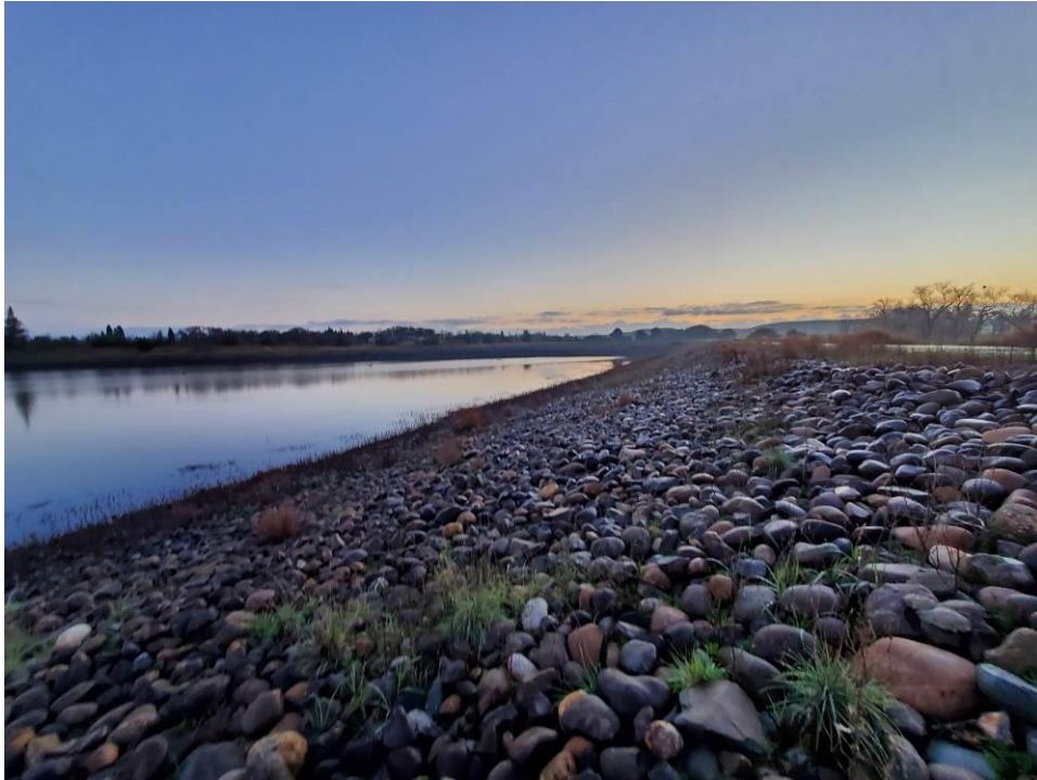
Photo 1: View of the south side upstream face of the dam at Reservoir No. 1 looking east.
