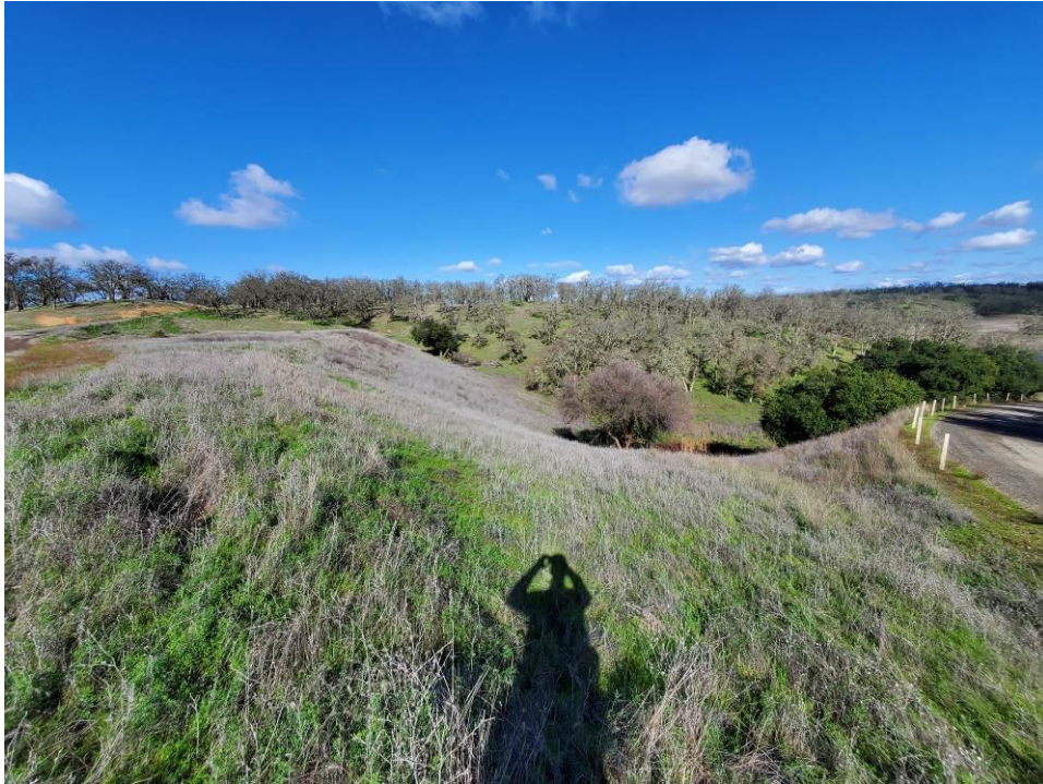
Photo 5: View of the downstream face of the North Dam from the right side looking towards the left.
