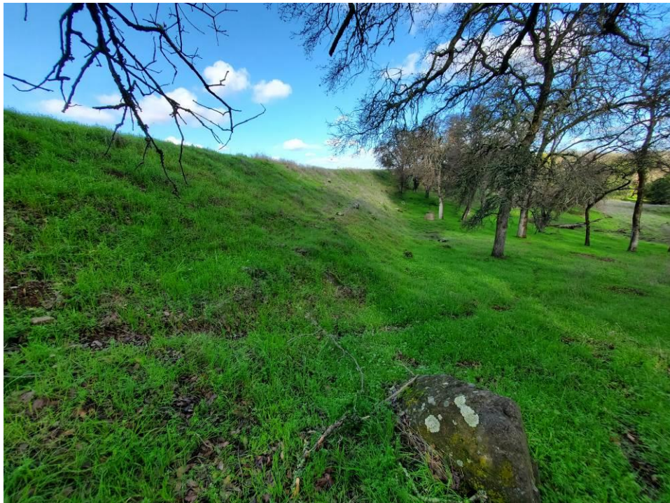
Photo 2: View of the downstream face of the South Dam from the right side looking towards the left.
