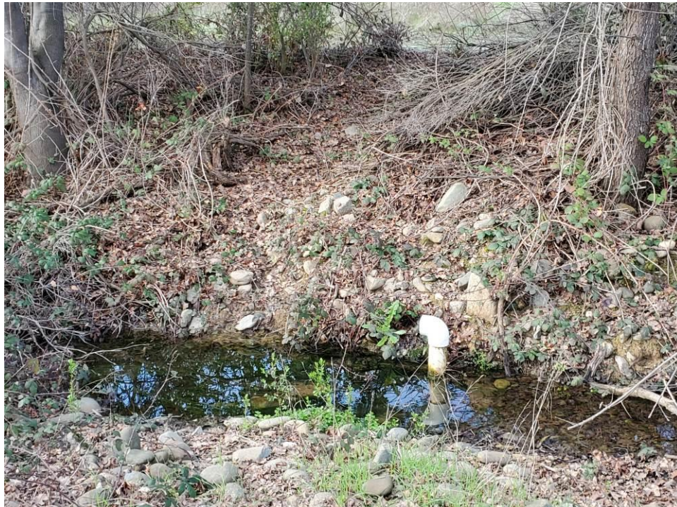
Photo 4: View of the seepage sump pump outfall in the ditch downstream of the toe of the dam.
