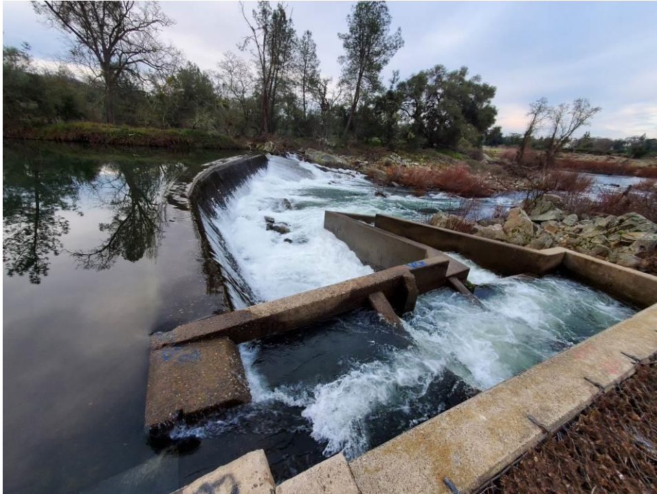
Photo 1: View of the North Dam from the right abutment looking towards the left.
