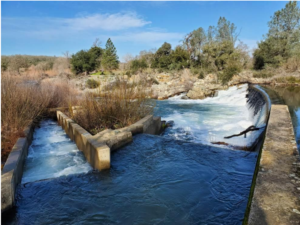
Photo 2: View of the South Dam from the left abutment looking towards the right.
