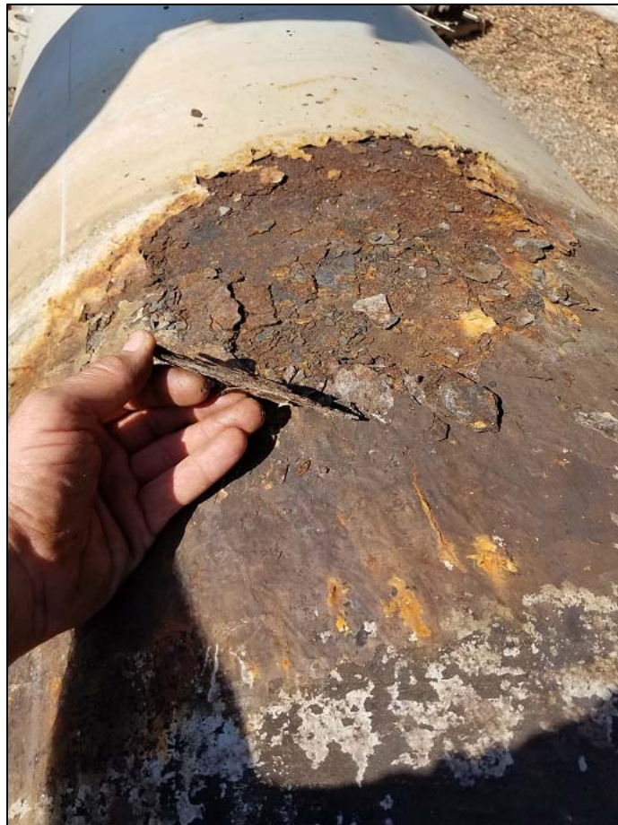
Corrosion of pipe column
