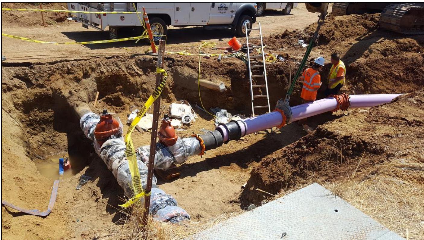
Installation of 12-inch recycled water pipeline running towards Murieta Gardens and commercial areas
